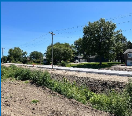
Power Poles to be Relocated
