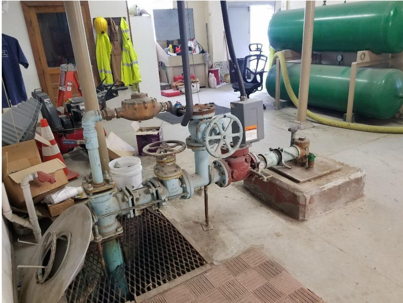
Existing Well No. 2 and Pump
