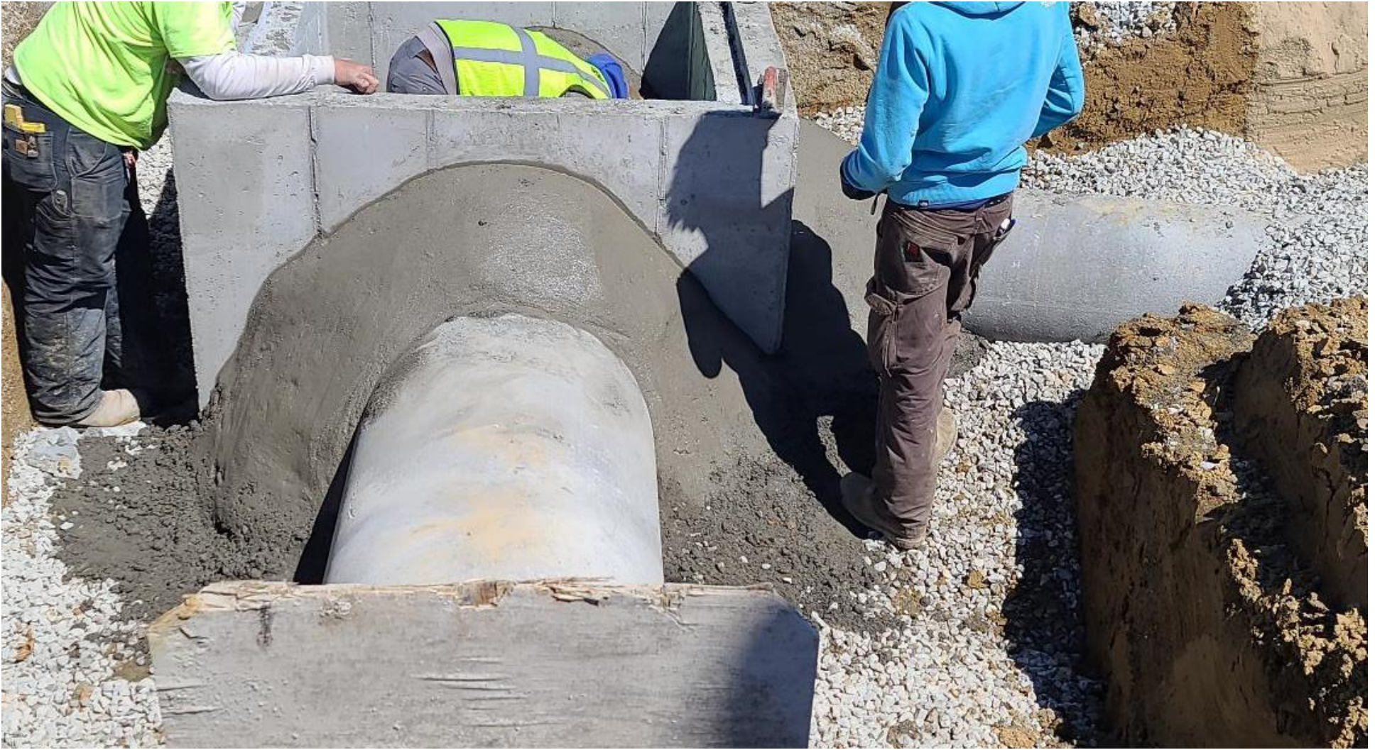
Storm Sewer Structure
