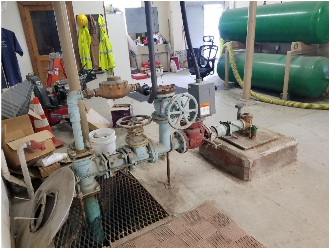
Existing Well No. 2 and Pump
